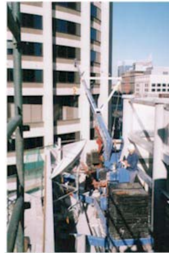
Lasco L10T working on Boulderstone Hornbrook site in Sydney CBD ... a new class of crane is created.
